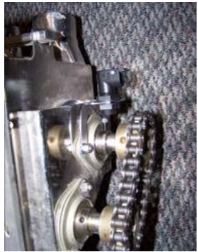
ROLLER STYLE SENSOR INSTALLATION
